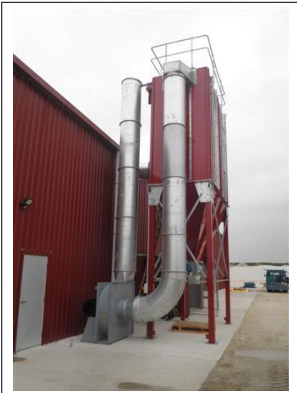
Southern Stone mineral dust Pulse Jet Filter, complete with rotary valve discharge into a skip
