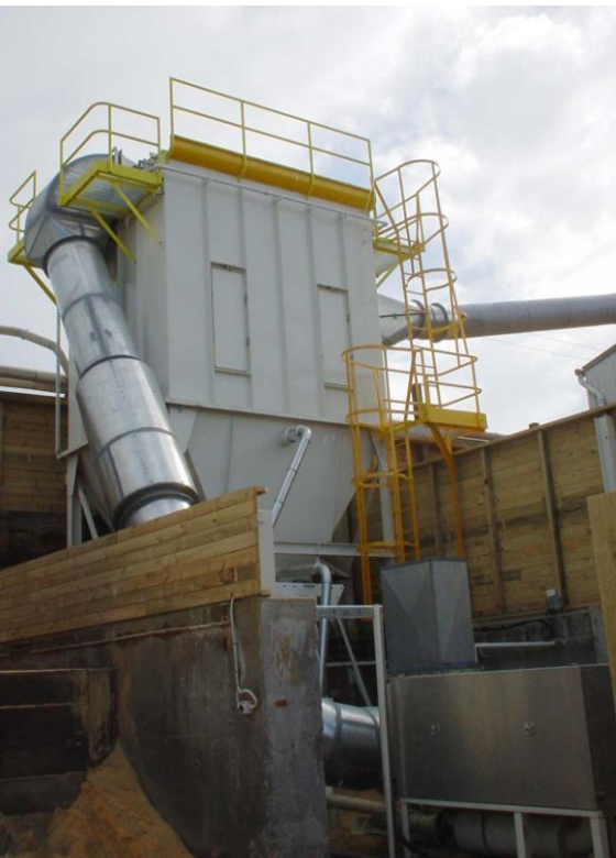
Taranaki Sawmills Pulse Jet Filter complete with high pressure rotary valve discharge, high pressure blower and blowline to silo
